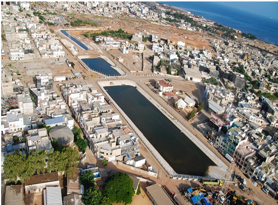
Reservoirs and drainage works built in Dakar to prevent flooding. © Agence de développement municipal (ADM)/PROGEP
